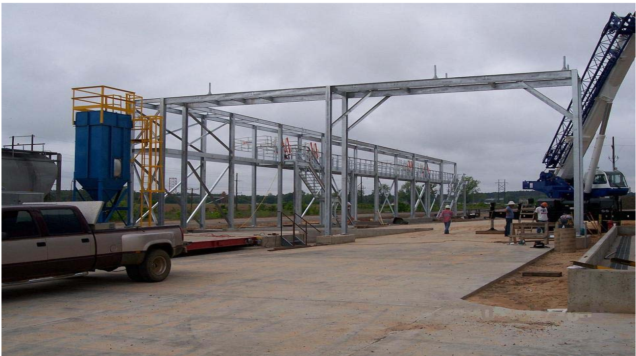
May 15, 2009 – The steel for the Pipe Rack and Loadout Platform has been erected.
