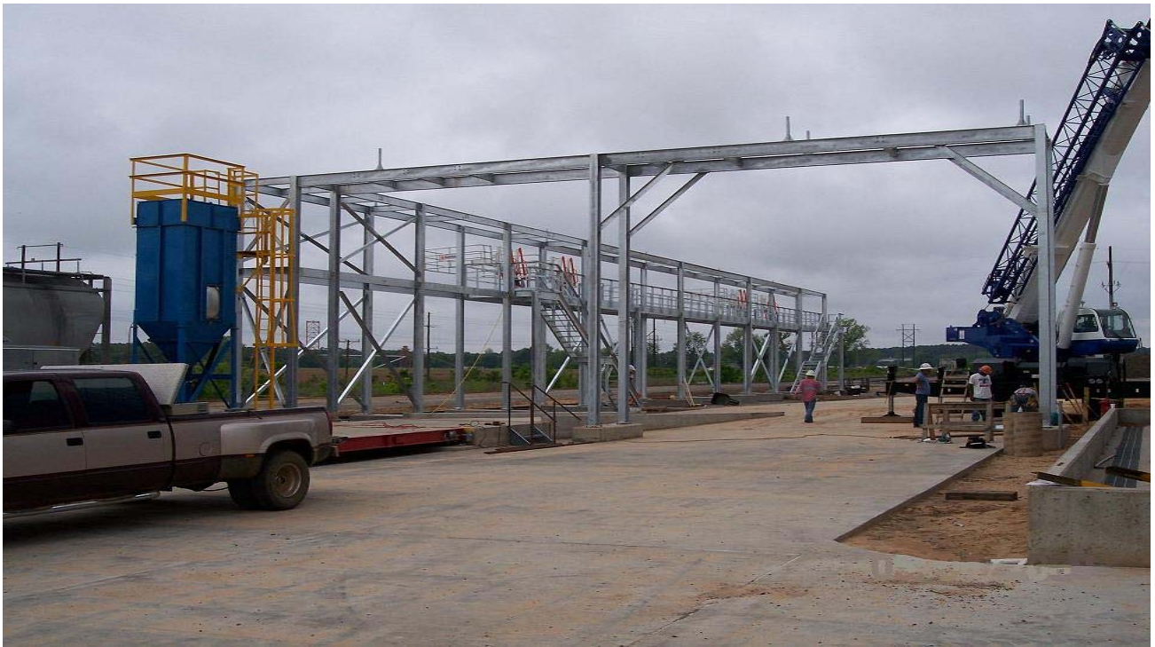
May 4, 2009 – The steel for the Pipe Rack and Loadout Platform has been erected.
