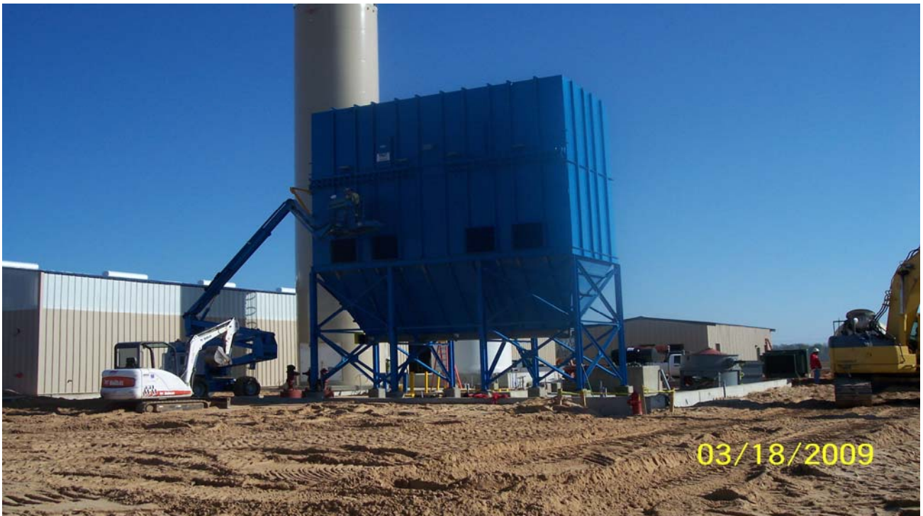
March 18, 2009 – Baghouse and Dust Collector for the Mill.
