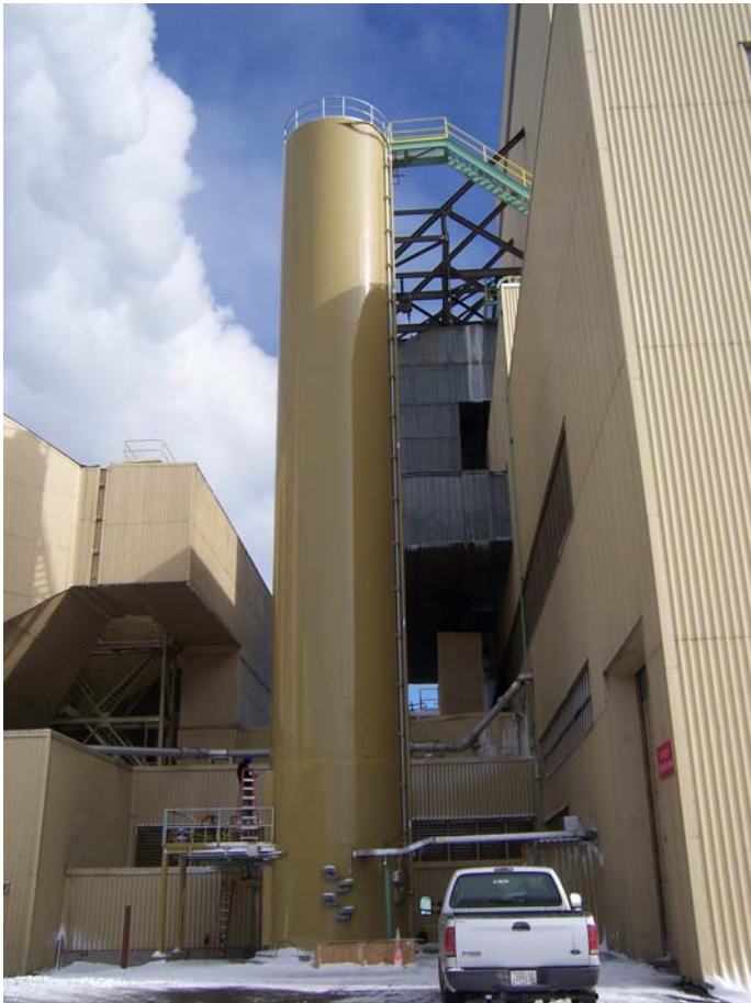
Figure 1. Edgewater Unit 5 ACI system silo.
