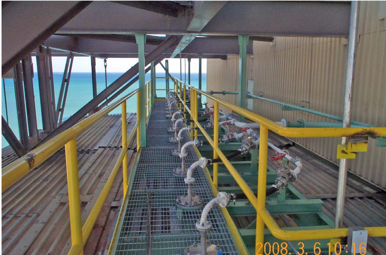
Figure 6. Sorbent injection manifold – economizer outlet.
