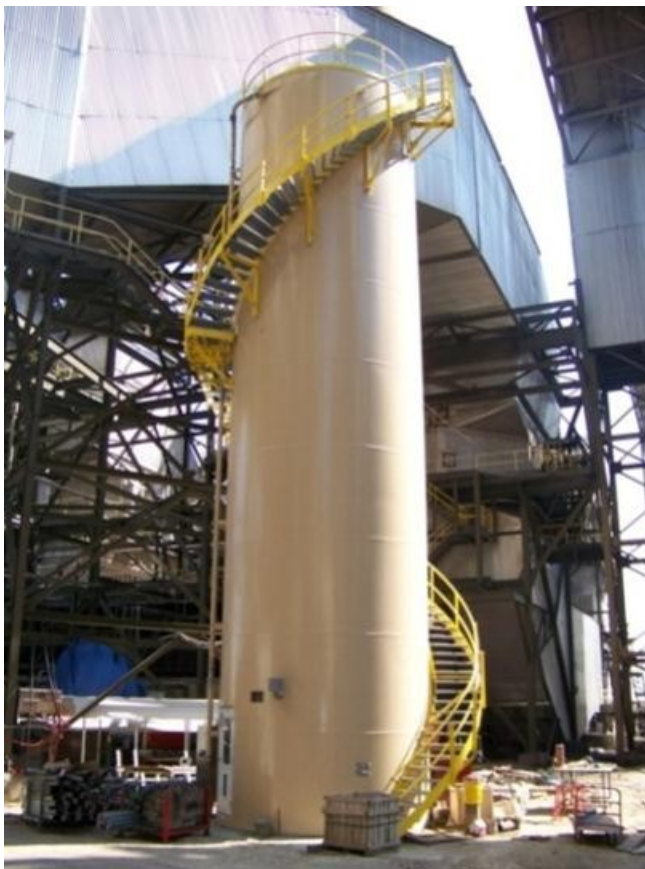
Figure 3. Example of a commercial ACI system (©ADA-ES 2010).
