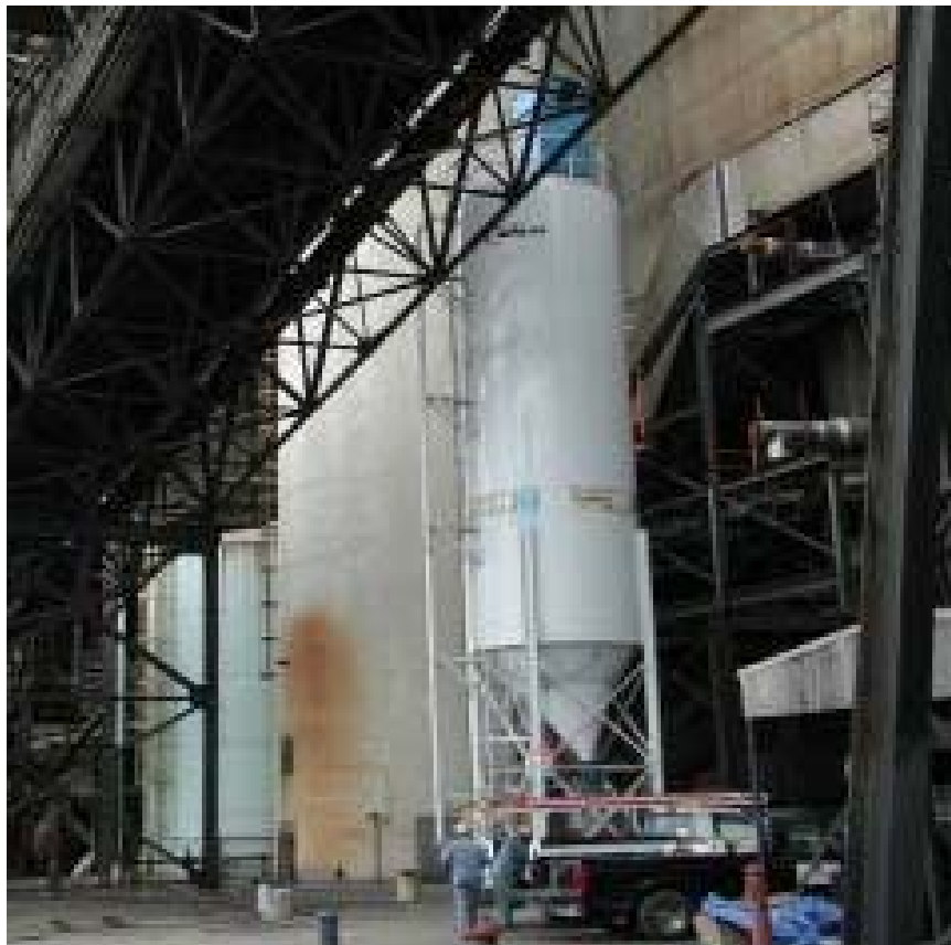
Figure 4. Carbon Injection Storage Silo and Feeder Trains Installed at Gaston, 2003–2004.
