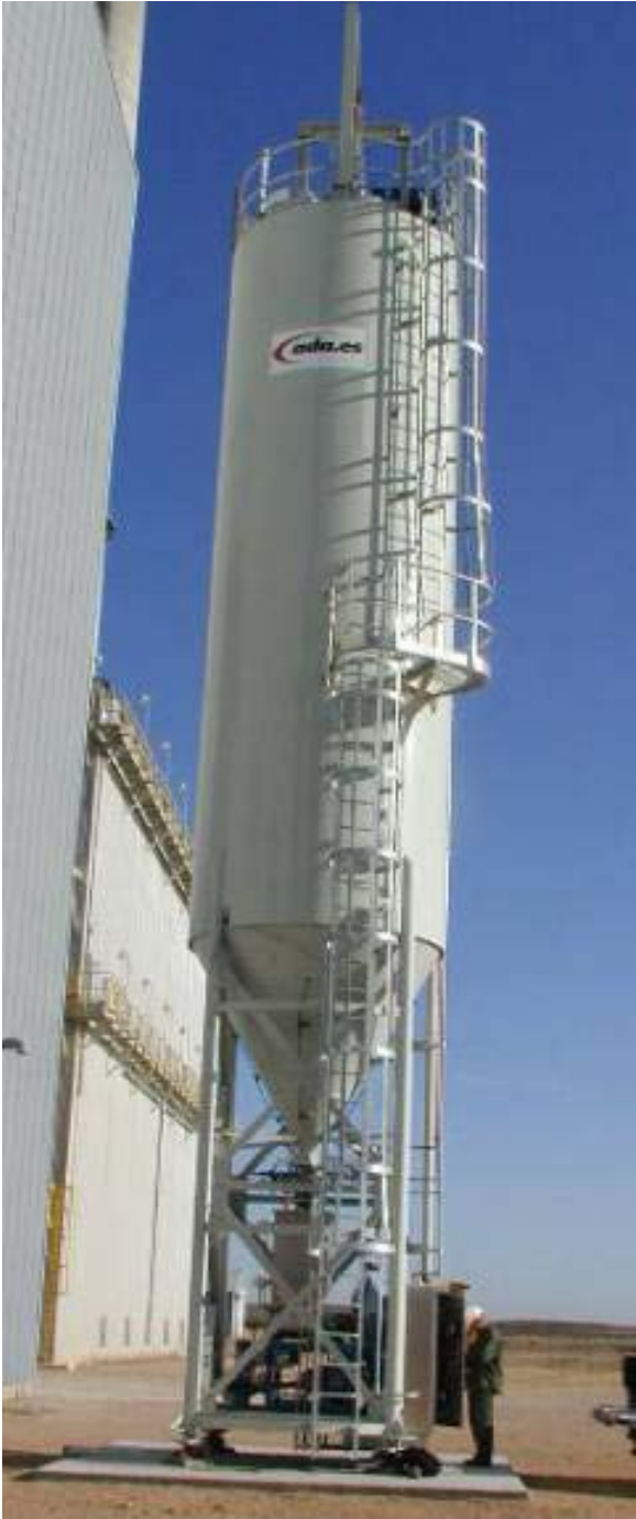
Figure 3. Photograph of Activated Carbon Injection System at Holcomb.
